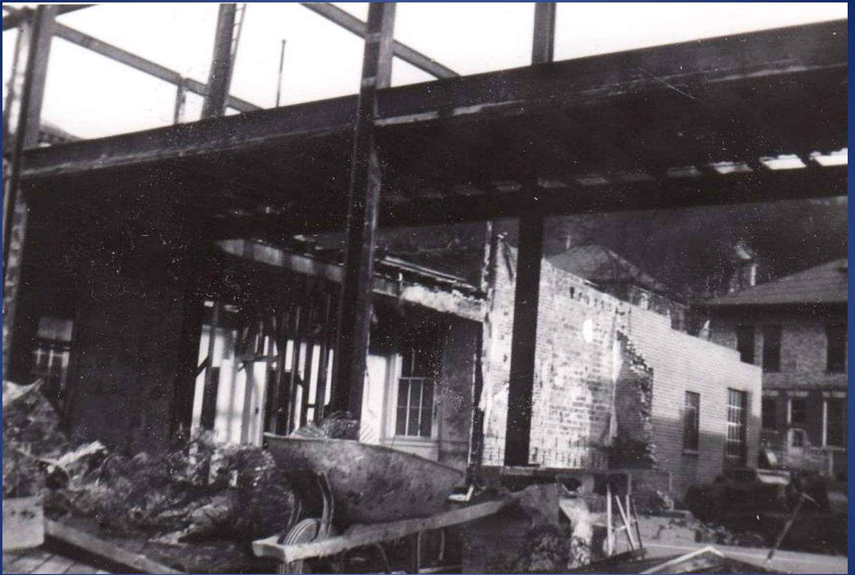
Results of Hinton High School Fire Notice Library Building on Ballengee Street
